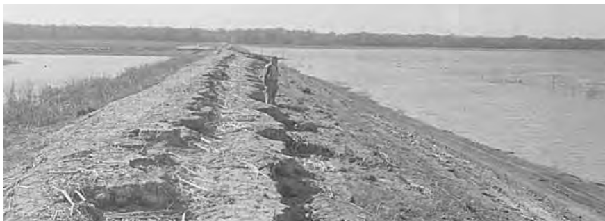
Flood damage 1961, from refuge files
